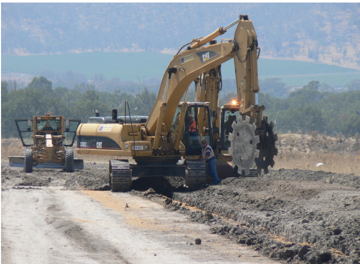
Above: Excavator fitted with a "Pizza Cutter" used to place and compact sand and earth backfill following laying of pipes.
