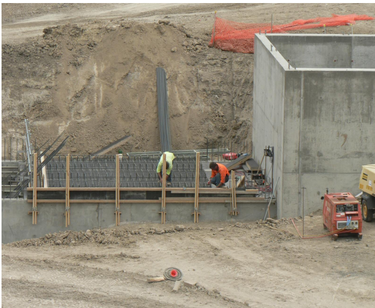
Above: Preparing for final concrete pour on top of the 'wet well' which provides the connection between channel and the pump station pumps
