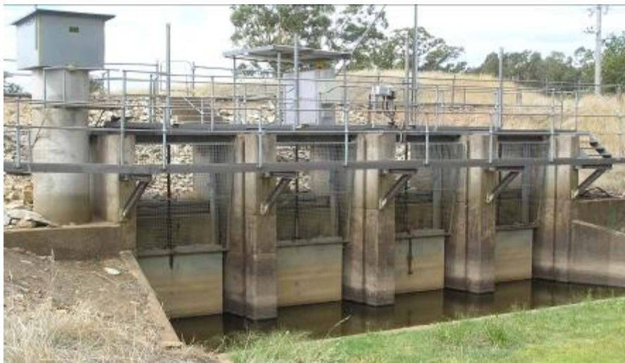
Figure 2: One of the existing structures that will receive new flow regulating gates and improved supervisory control and data acquisition (S.C.A.D.A) equipment to enable the remote control and monitoring of water levels and flows.
