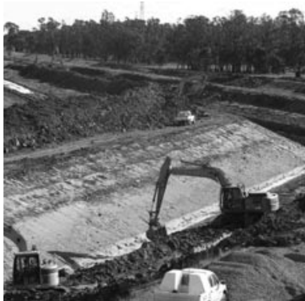
Works commence on the outlet channel. The channel will be deepened to allow water to flow from the Broken River to the dam wall and into the proposed new pumping station.
