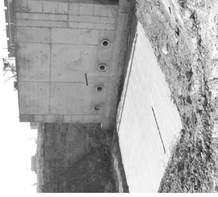
The building and civil construction phase for the pump station is also nearing completion, with all pump and pipework installed and the electrical cable, switchboards and control panel installation in progress.
